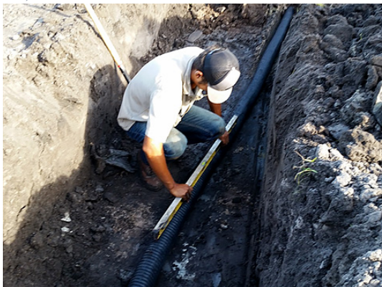
Figure 7. Installing subsurface irrigation drain tile to replace less efficient seepage irrigation (Source: SJRWMD, http://www.sjrwmd.com/permitting/regulatorynews/archive/2016-04/ )
